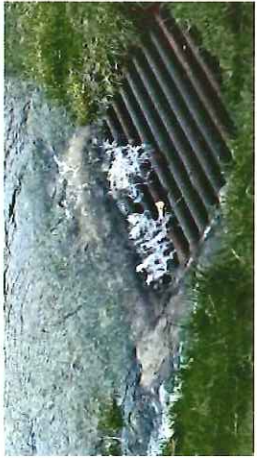
An overloaded storm sewer
